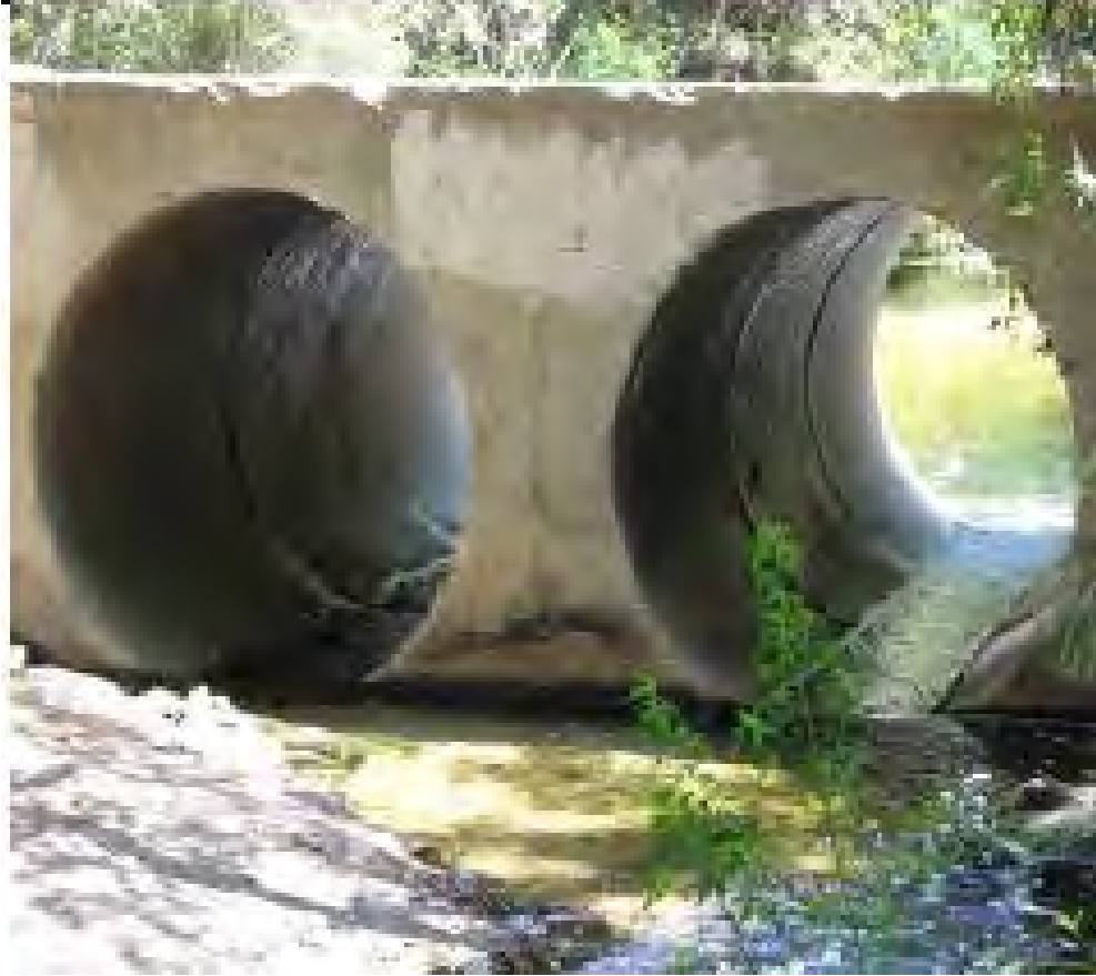
1 2 Figure 3.1-2 LV1, Craggs Road Culvert (Picture taken while looking upstream toward the outlet of 3 the culvert)
