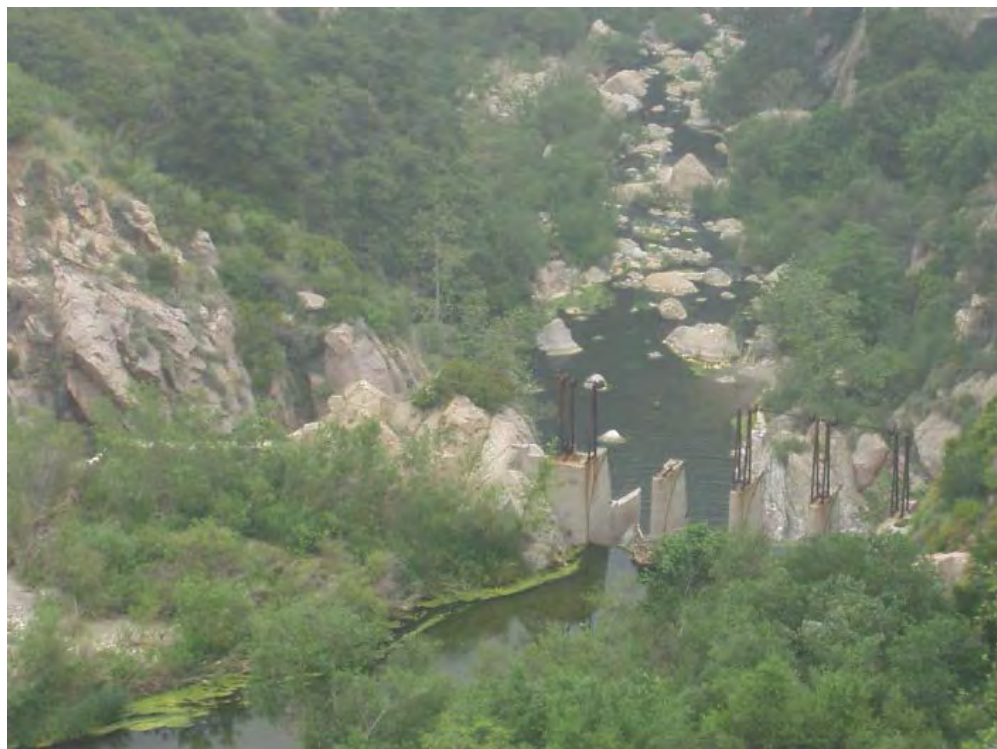
Clockwise from left: View of the downstream face of the dam, left and right abutments, and spillway. View of the upstream face and crest of the dam. Sediment has deposited on the upstream face almost to the top. View of the upstream side of the spillway.
