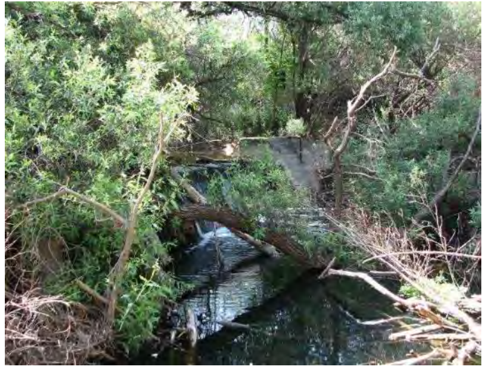
Photo 4.4-7 - LV2 Check Dam
